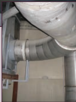
A new airflow system comprised of stainless steel tubing redirects air emitted from three extrusion lines into odor control units from APP.
