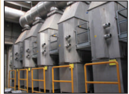
These APP units (installed at a Nestlé Purina facility) have fans with three different speeds, based on temperature of the dryer air coming from the extrusion lines. Each unit has a cooling system, too.
