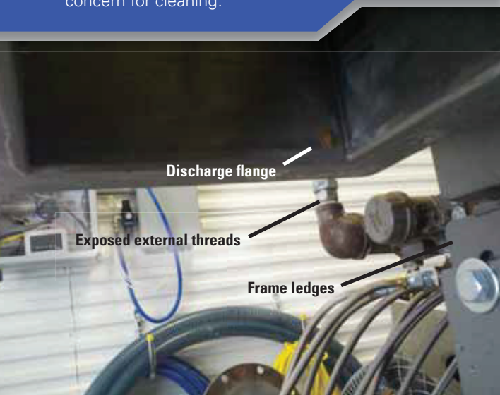
Figure 2. ADP Discharge Flange – Highlighted areas of concern for cleaning.
