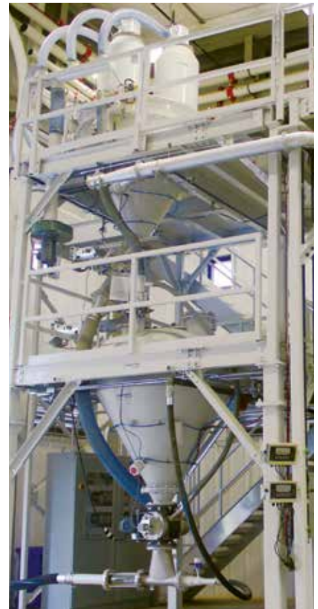
Photo 2 - Dense phase conveying system
