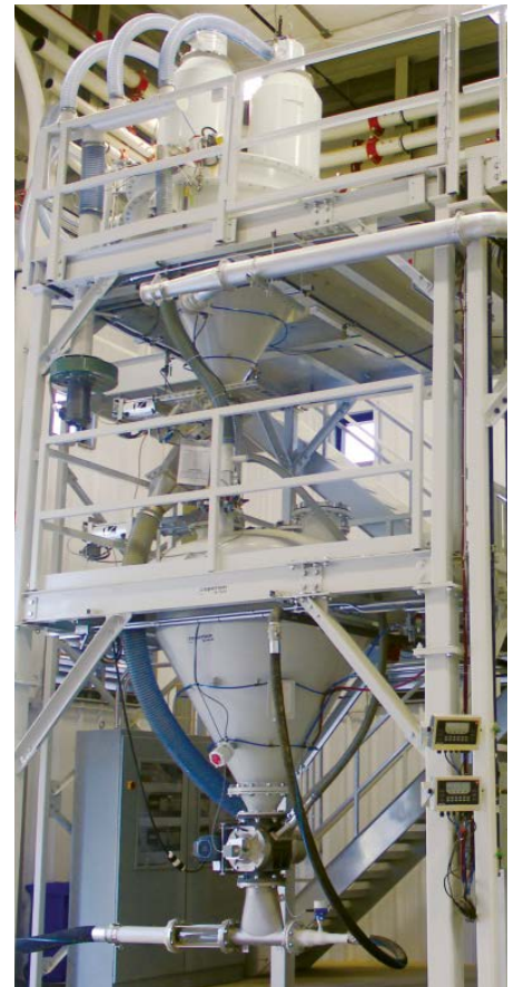
Photo 2 - Dense phase conveying system
