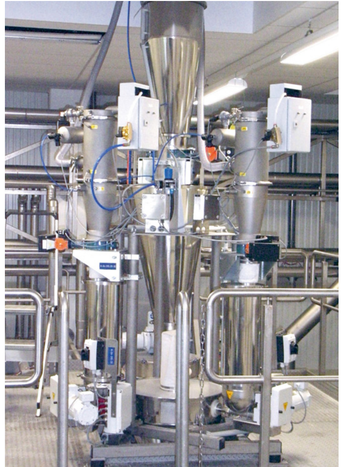
Fig. 4: Gain-in-Weight Batching system in a food application
