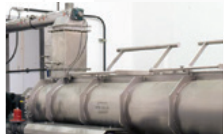
The AVT system for steam & fines suppression from Dual Cylinder, no venting of dust or steam to atmosphere.
